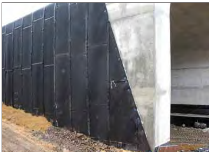
Obr. 11 Ochrana hydroizolace recyklátem pryže ELTEC Fig. 11 Protection of the waterproofing with ELTEC recycled rubber plates
