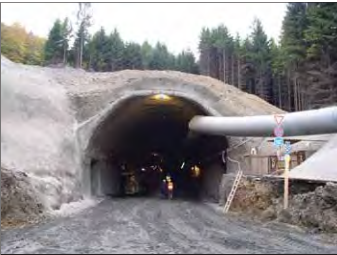
Obr. 14 Ražba tunelu Malá Huba pod provizorní klenbou Fig. 14 Driving the Malá Huba tunnel under the temporary vault
