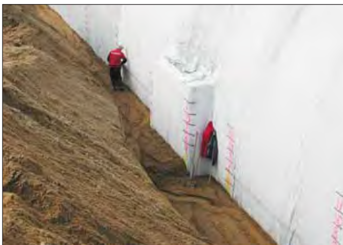
Obr. 2 Postupné obsypávání tunelu podle rysek na geotextilii Fig. 2 Gradual backfilling of the tunnel according to marks on the geotextile
