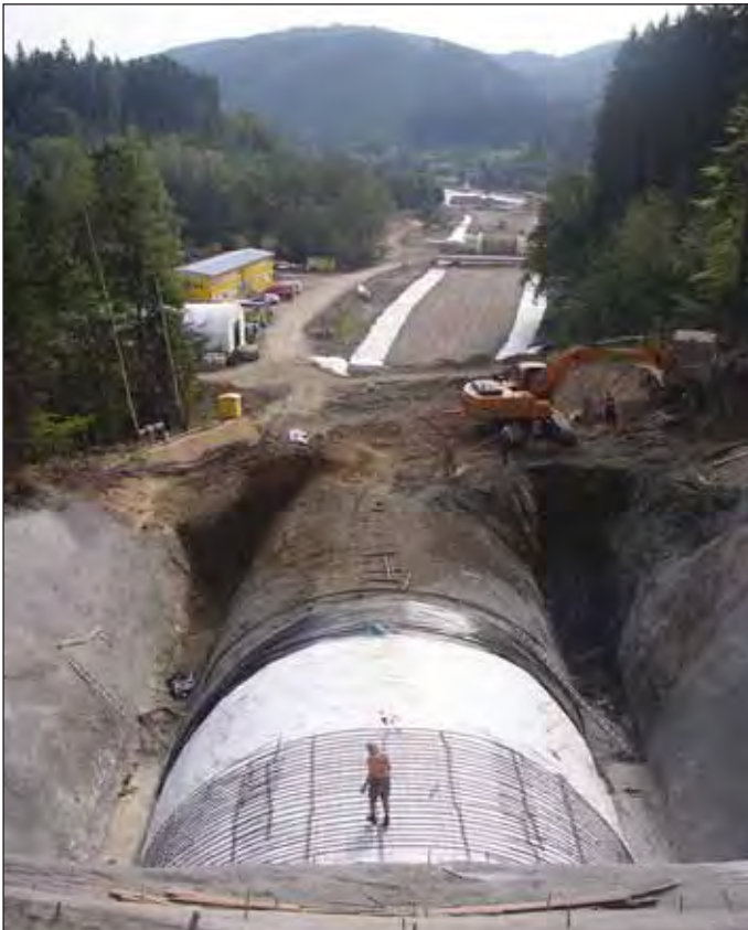
Obr. 13 Tvarování horniny do profilu klenby Fig. 13 Moulding of ground into the shape of a vault
