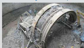
Znižený Perforex. Destroyed Perforex.
