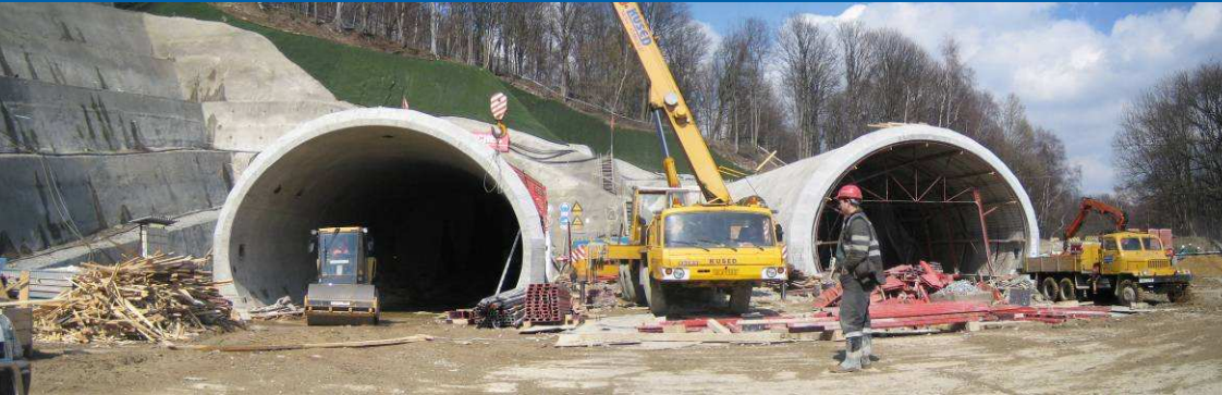
■ Highway tunnel Libouhec – highway D8 Prague/Dresden
